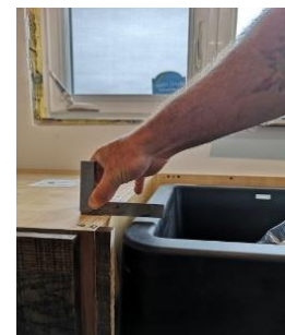
This sink is too low.
